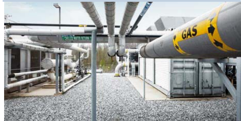
BMW Spartanburg Plant Methane gas project
